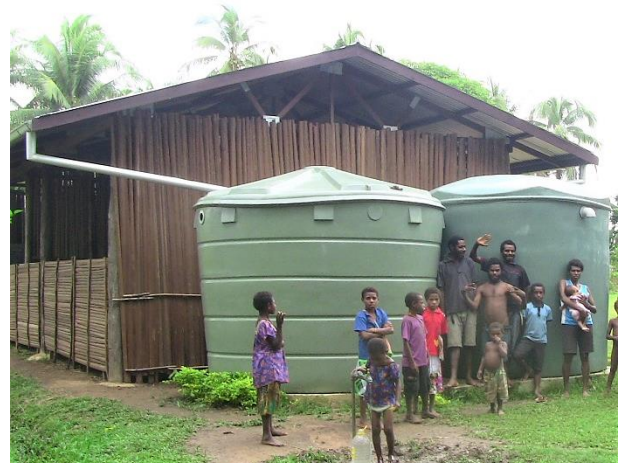
Water tanks installed on a PIM classroom
